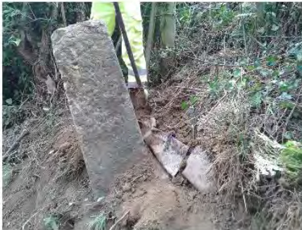
A long steel sheet behind the Stone was pressing against it; this had to be cut and removed.
