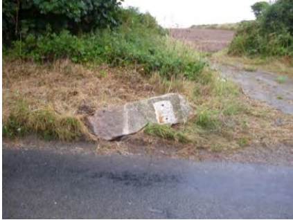
Knocked over and with plates missing in July 2018 Photos: Ian Thompson
