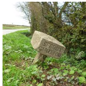
SX057721 B3266 6.11.17 After most recent damage. Capstone replaced by Cormac but not fixed. Pillar at an alarming angle.
